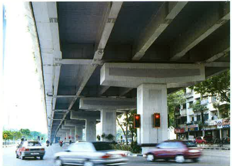
RT3 floodlights as soffit lighting at elevated highway along Jalan Tun Abdul Razak.
