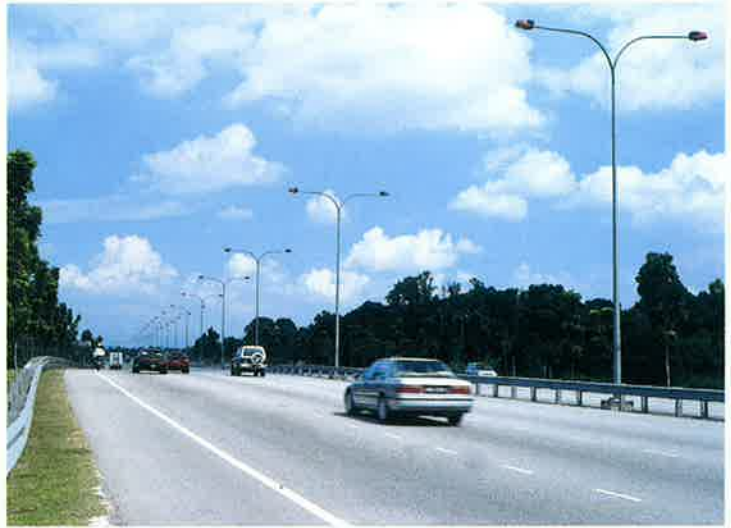
Z2 lanterns installed at the Cheras-Kajang Highway, Kuala Lumpur
